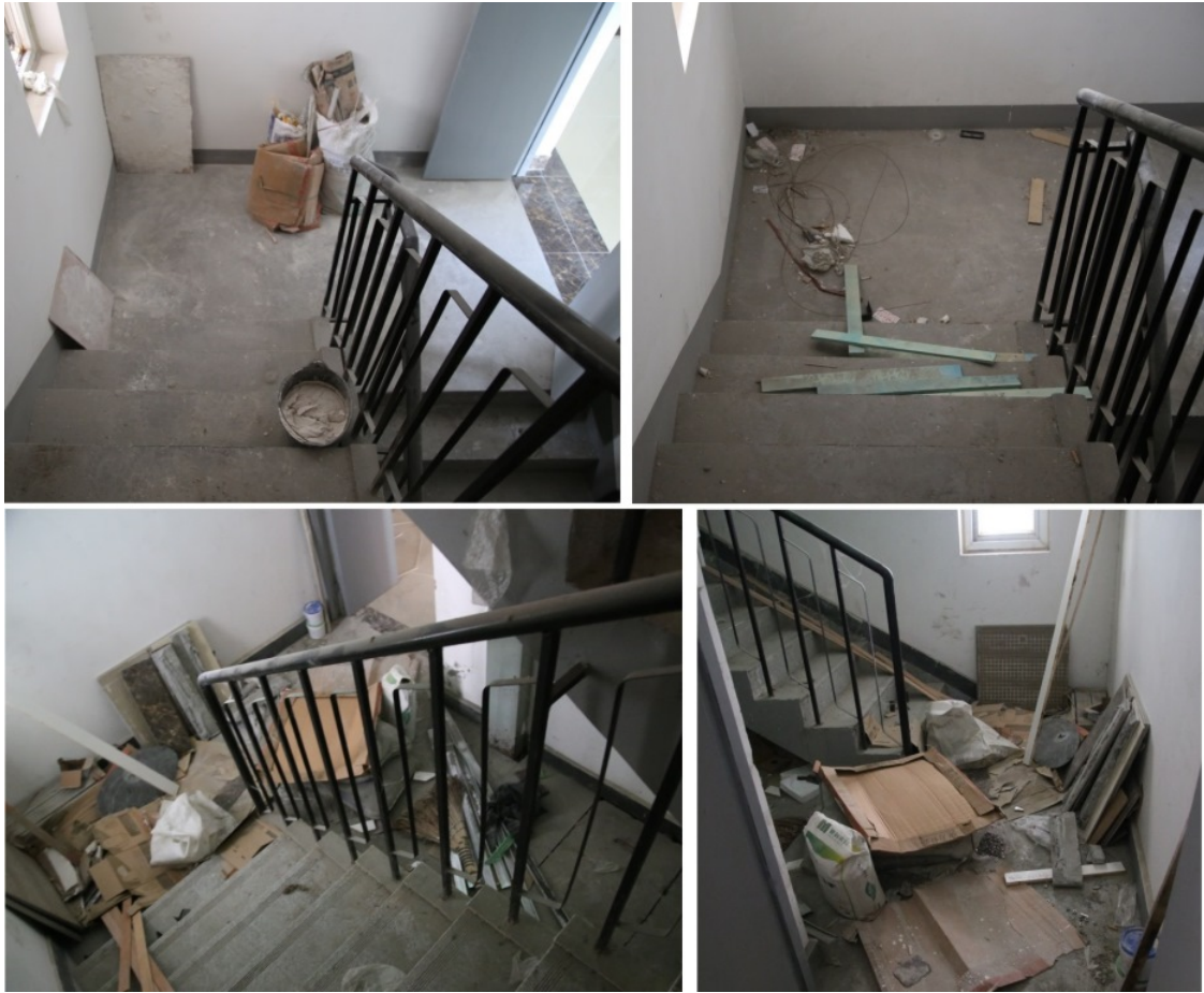
Figure 4: The stairs, which are supposed to also serve as emergency exit, were full of junk and garbage. Lots of things were sharp and dangerous. Walking upstairs or downstairs was sort of a Russian Roulette, wondering each time whether we get hurt or not. The scary thought was of getting a large cut on the 8th or 9th floor, which were 8-9 flights away from people.
