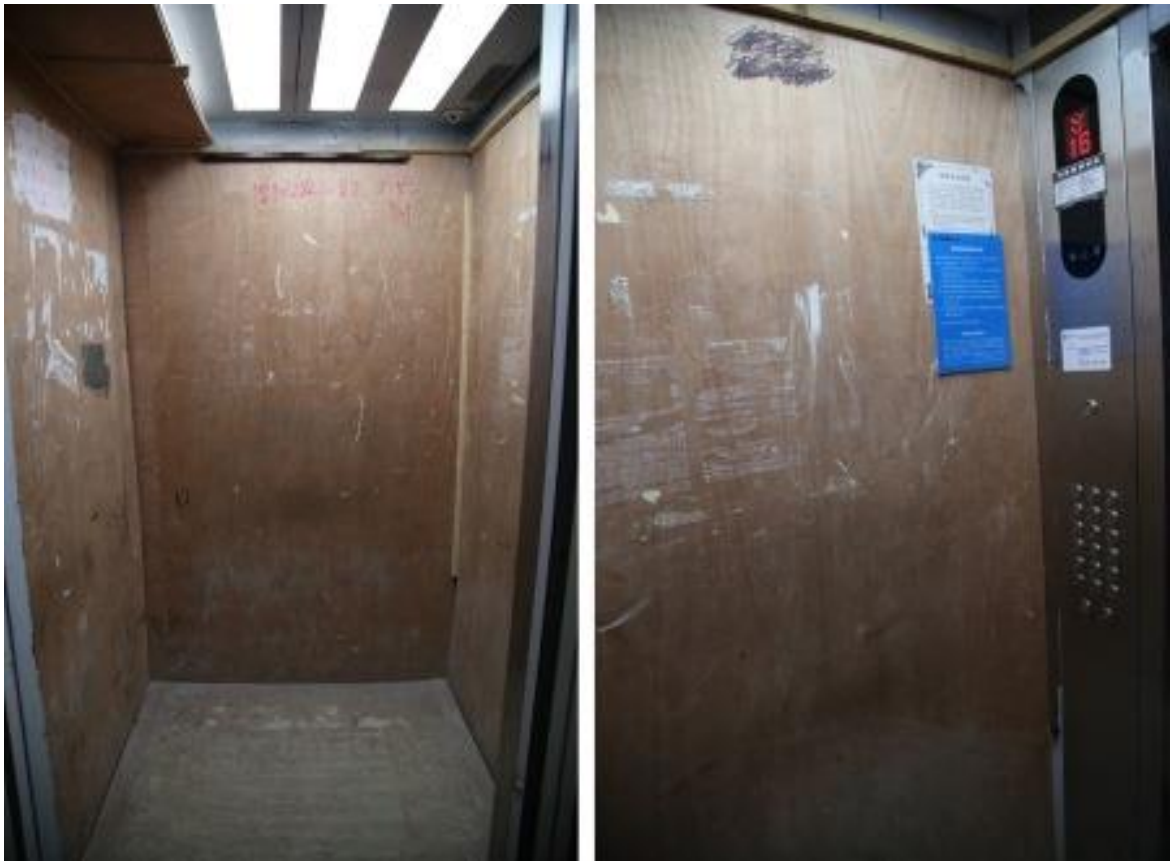
Figure 3: Of the two elevators, only one was working. It was small, the walls were covered with plywood full of splinters. The building was supposed to be for foreign experts, yet the signs were all in Chinese. Often the single working elevator was used by the construction workers and we had to use stairs.
