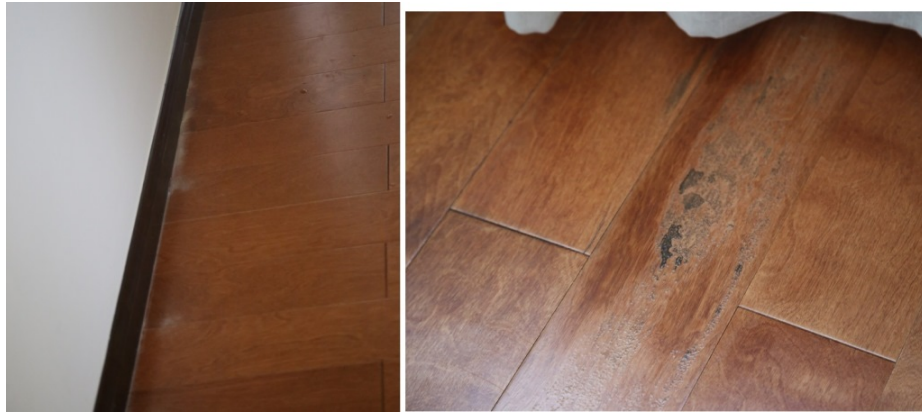
Figure 7: The dry wall was not properly sealed and white powdery stuff fell on the floor every day accumulating along the baseboards. The flooring was laminate with the cover coming off. Both the white dust and the laminate cover were chemicals, their exact chemical makeup unknown I could not even guess how harmful they might be, but http://news.bbc.co.uk/2/hi/8326621.stm may give an idea.
