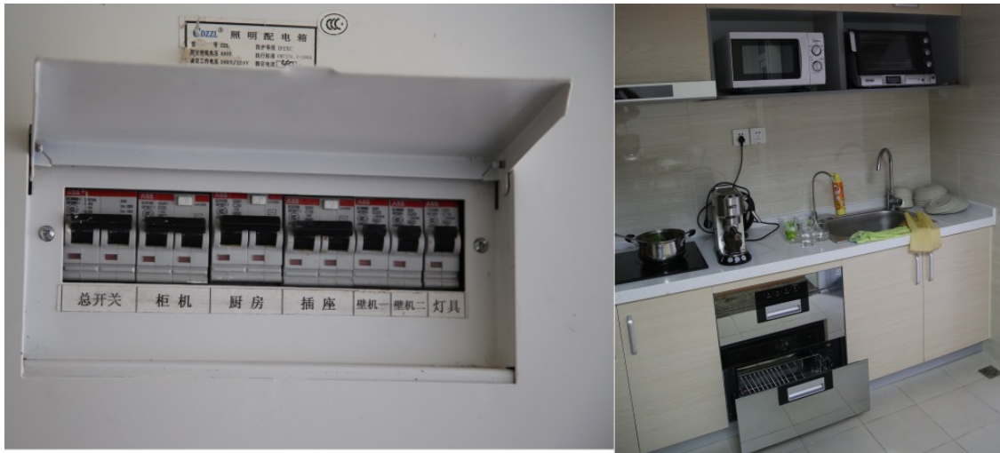
Figure 9: On the left is the apartment circuit breaker panel. On the right are the kitchen appliances besides the fridge, all were on the same circuit, together with the washer/drier and the heater.
