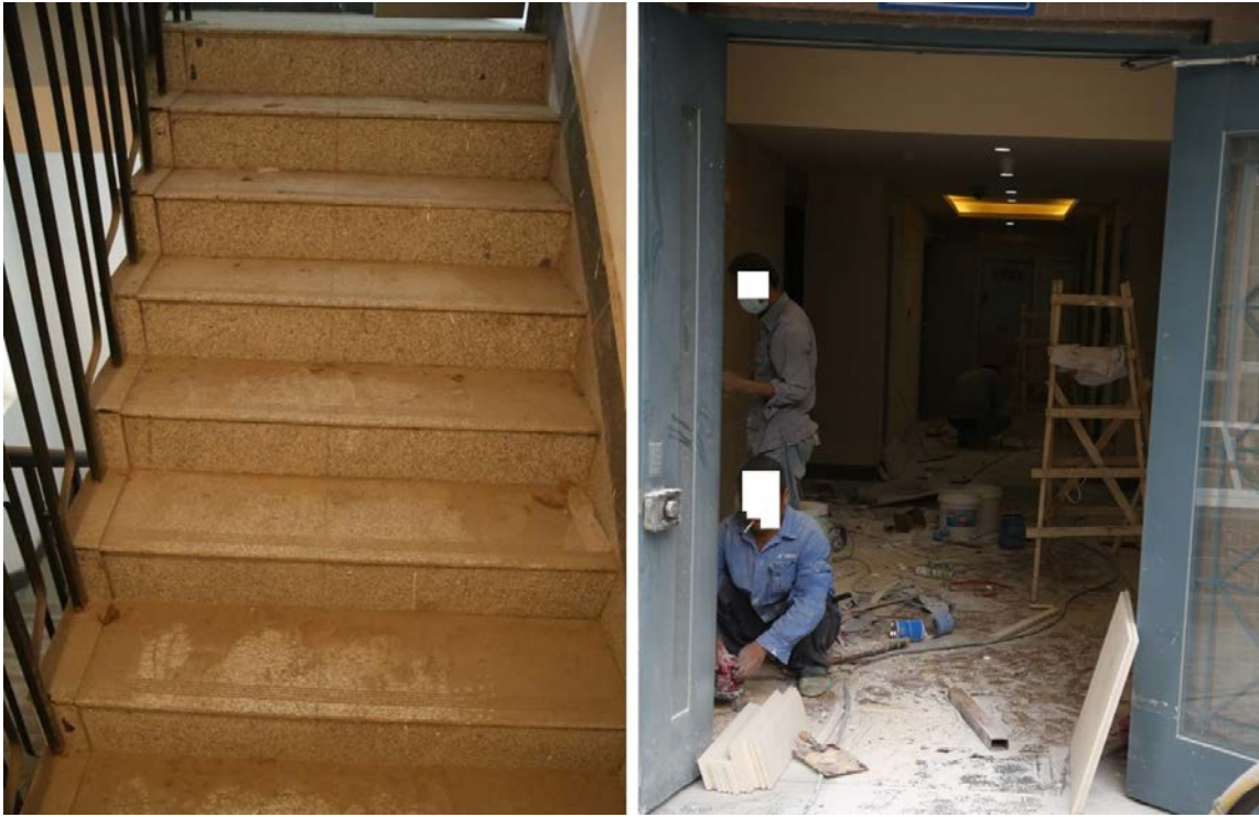
Figure 5: The few flights free of junk were covered with small loose particles making them slippery and dangerous to run on in case of an emergency. The picture of the lobby was taken on October 8, 2015.
